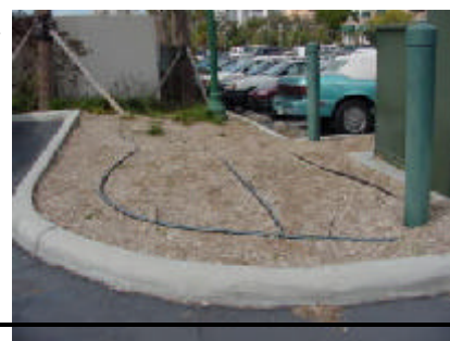
Water supply lines
